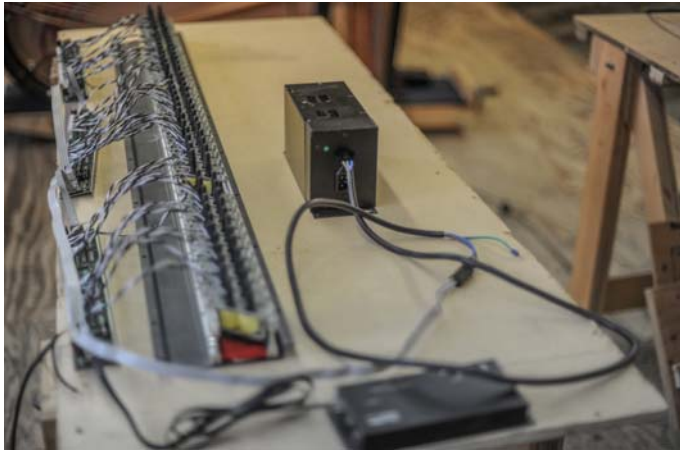
Illustration 130 - Connecting 40v power to driver boards
