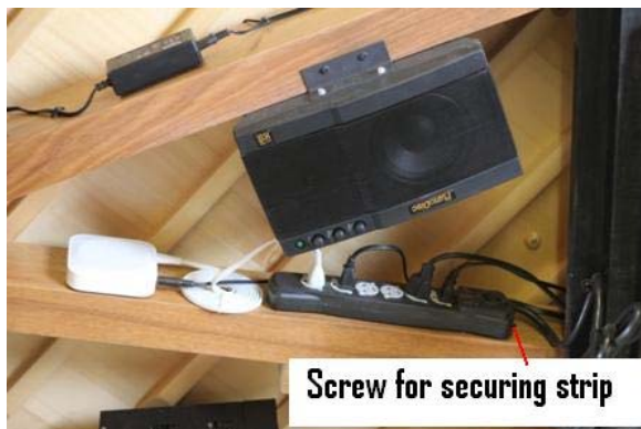
Illustration 137 - power strip mounted to beam
