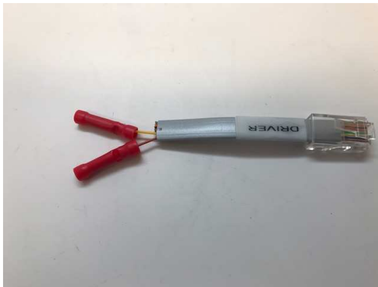
Butt splice terminals installed
